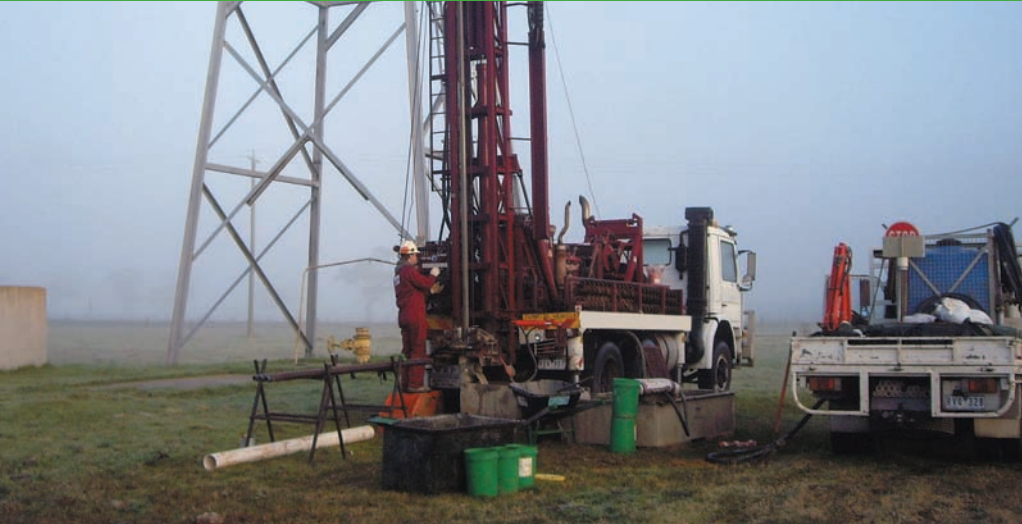
Groundwater bore installation into the Boisdale Formation aquifer (Warruk Sand Member), West Gippsland, Victoria.
