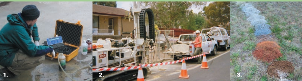
1. Groundwater sampling (Colac, Victoria); 2. Off-site groundwater bore installation (Stawell, Victoria); 3. Air hammer returns (concrete, topsoil and red clay over basalt) (Ballan, Victoria).
