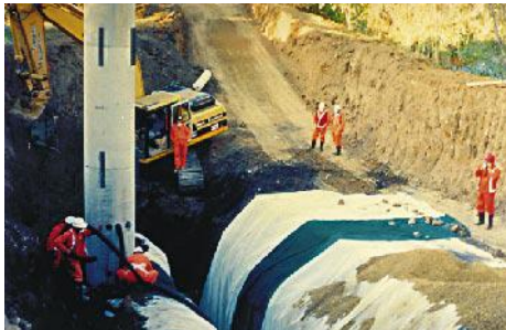
Inserting a sump during the construction of a cut-off trench to prevent contamination from an old gas works from reaching a river.
