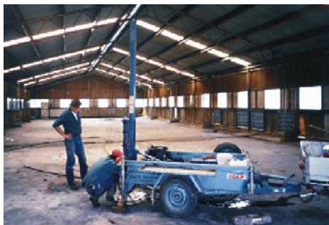
A Mark I light-weight drilling rig being used to core through a concrete floor inside a warehouse.
