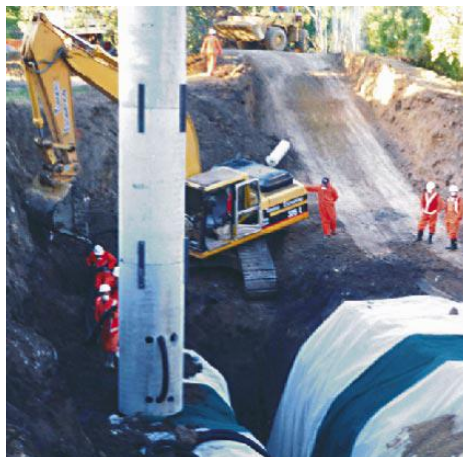
A cut-off trench is constructed to prevent contamination from an old gas works from reaching a river.
